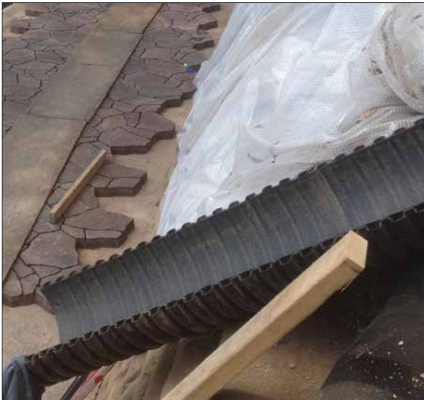
» They used 24" PVC chutes bolted together to send materials like sand, stone and plant plugs down to the work area.
